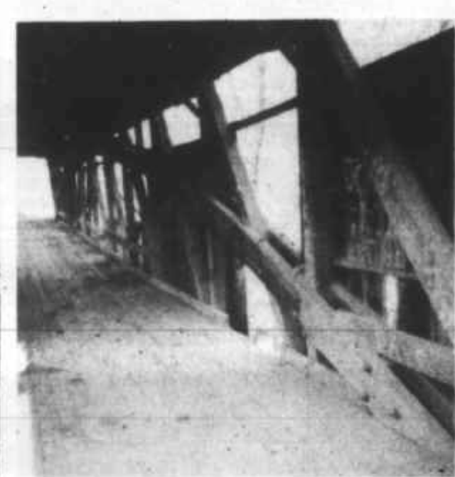
photo shows the bridge in its current dilapidated condition, while the right photo shows some of the interior wooden structure.
